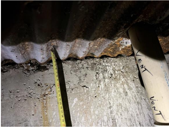
Item S1 – Frost and deteriorating metal deck over utility tunnel located around perimeter of Main Level Classroom space.
