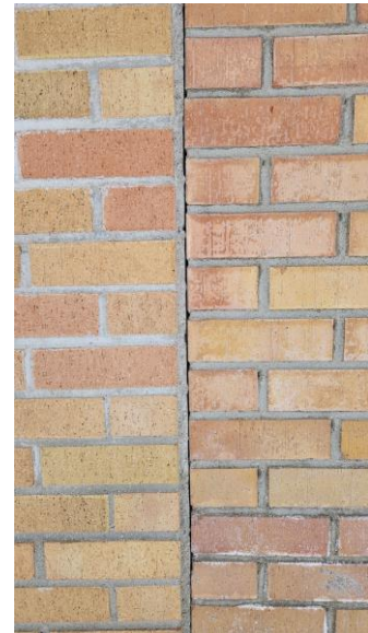
Item S7 – Masonry joint on north wall of Room 122. Variation in brick and differential movement can be seen between left wall (Room 122) and right wall (Stair 121).
