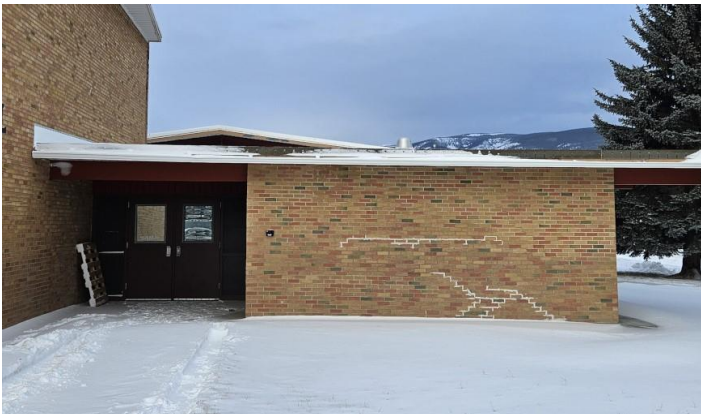
Item S7 – East Wall of Room 122. Damaged and subsequently repaired mortar joints can be seen.
