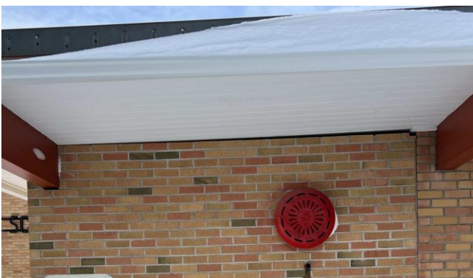
Item S7 – Top of Room 122 North wall. Gap between top of wall and roof deck varies in depth.
