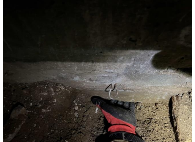
Item S1 – Typical Main Level Foundation wall base. No continuous wall footing present.
