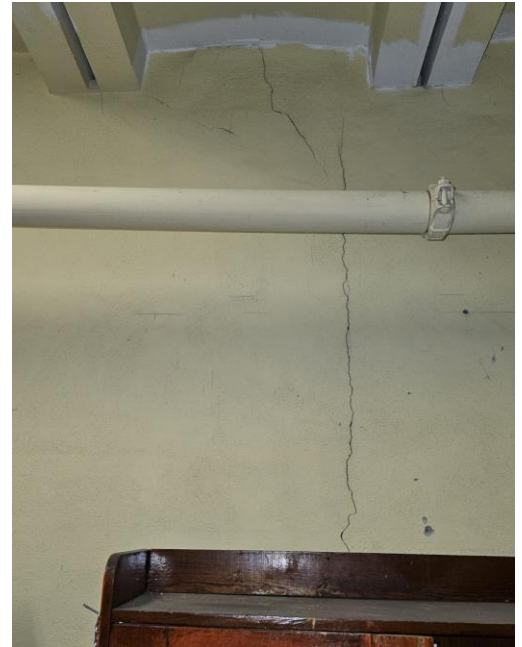
Item S5 – Typical foundation wall crack over cabinet in room 011
